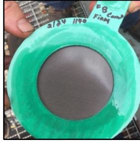
Figure 10. Compressor inboard bearing approved second (confirmation) inspection 2/24/18 11:40AM
